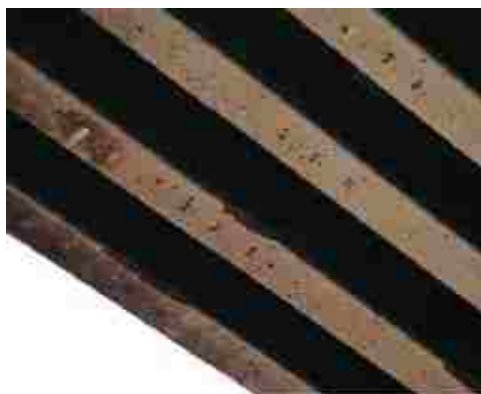
Figure 6.8 Damaged concrete located at the bottom of the girders (location which was closest to heat source) (Aspire, Spring 2008)
