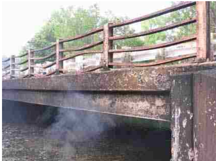
Figure 2.7 Damaged Norwalk Bridge near Ridgefield, Connecticut due to an overturned gasoline tanker (FHWA, 2007)
